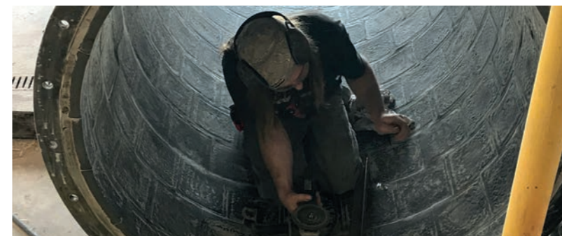
Kalenborn special ducts and bends for a biosolids recycling plant: straight ABRESIST ducts and bends with KALOCER and KALCRET
