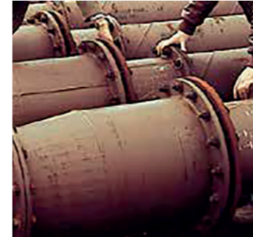
Expansion joint in a hydraulic ash line
