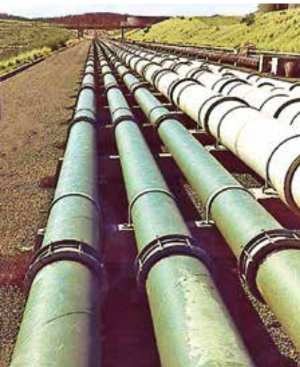
Wear protection for hydraulic and pneumatic pipes
