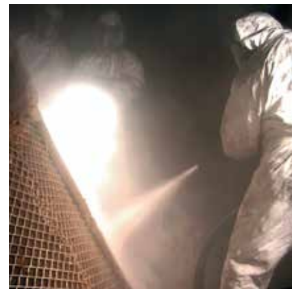
When particularly high dust loads occur, the waste gas ducts are protected by KALCRET hard compound or KALMETALL hard overlay welding.
