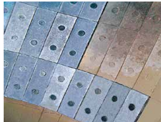
Lining of an infed coal pulverizer with KALCAST.
