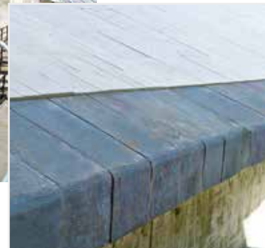
Discharge edge of a coke loading bay the KALCAST hard cast components are fixed mechanically
