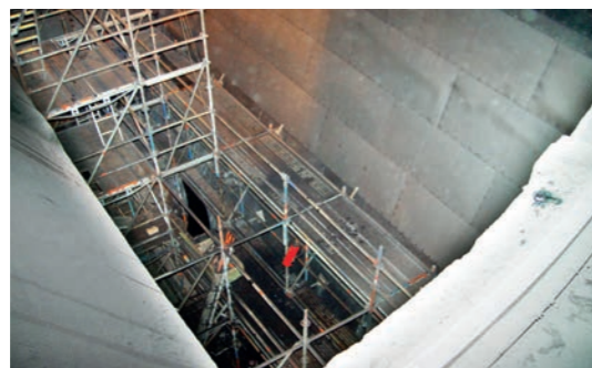
KALEN lining in the upper part of a fine coal bunker.
