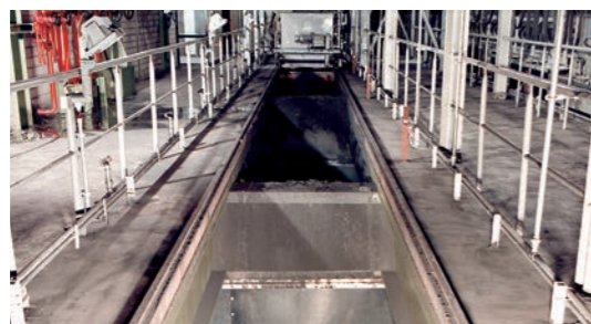
KALEN lining installed in a large German coal-fired power station. The material in the bunker is fine coal.
