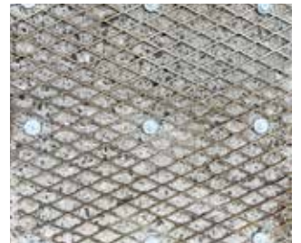
Attachment of wire mesh to concrete – distance to the wall to be lined: 5 mm / 0.19 inches
