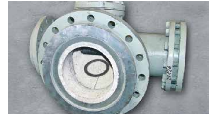
Pipe diverter in pneumatic pipe lined with KALCOR
