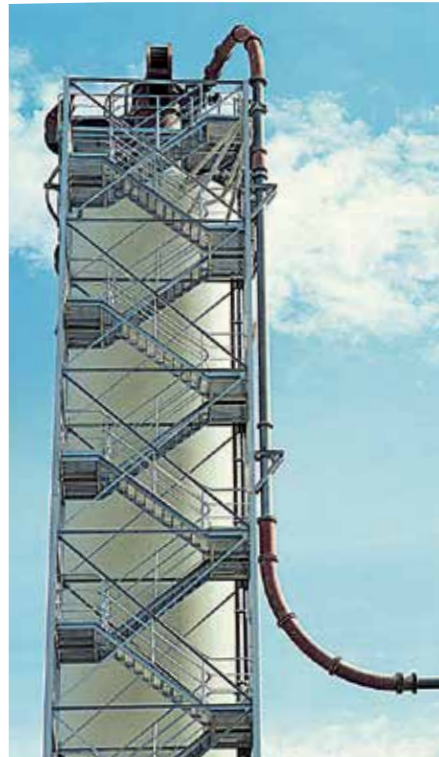
Transport pipe to the cement silos; the bends are protected by ABRESIST
