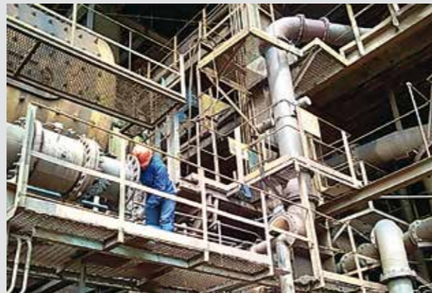
In Brazil the rubber lining in the pipe from the grinding mill to the classifying of the iron ore failed after a short time. These pipes are now lined with KALCOR zirconium corundum.
