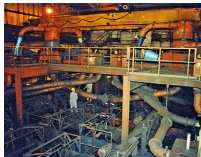
Hydraulic conveying pipes integrated in a coal preparation plant in North America. The pipes have been lined with ABRESIST. In this case they reach service cycles of more than 20 years.
