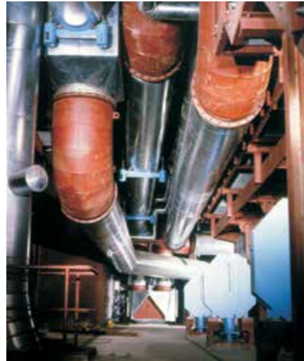
A typical application in power plants is pulverized fuel piping.
