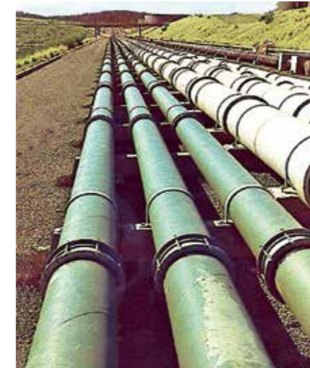
Wear protection for hydraulic and pneumatic pipes
