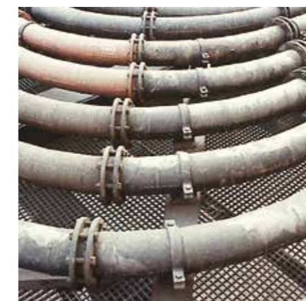
Extended service life of plant components
