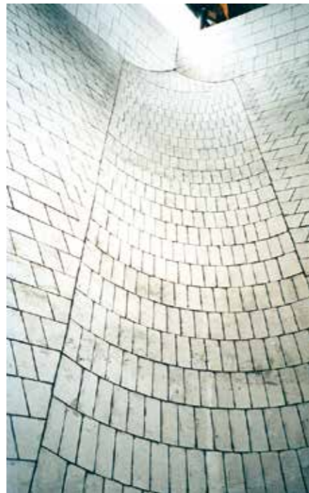
Bunkers for blast furnace charging are effectively lined with KALOCER
