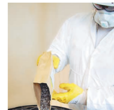
Add fibre components slowly and continuously and mix dry for about 1 minute
