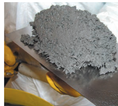
The stiff / plastic KALCRET compound (X) to be applied by trowelling with the aid of simple bricklayer tools
