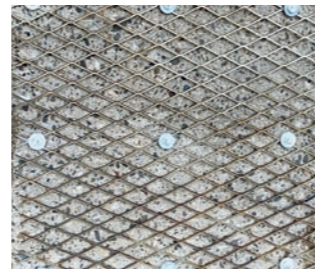
Attachment of wire mesh to concrete – distance to the wall to be lined: 5 mm / 0.19 inches
