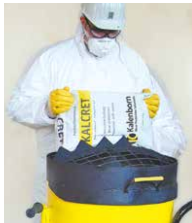
Material feeding into the forced circulation mixer
