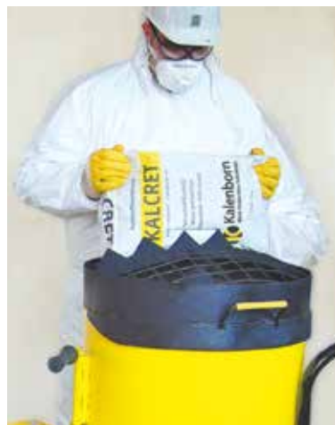
Material feeding into the forced circulation mixer
