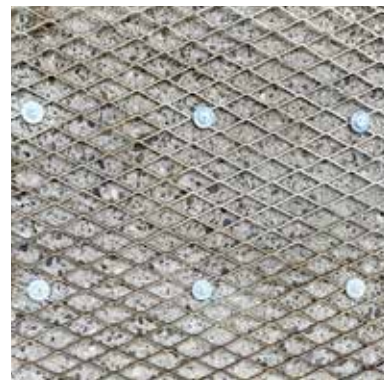
Attachment of wire mesh to concrete – distance to the wall to be lined: 5 mm / 0.19 inches
