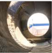
A pre-separator in the flue gas cleaning
